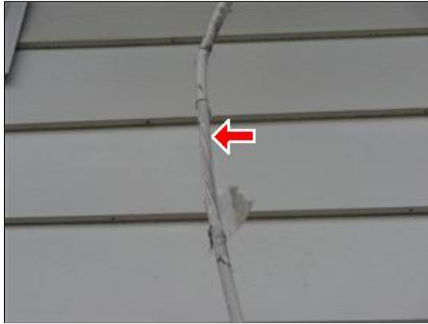
7.0 Picture 1 wires frayed here
