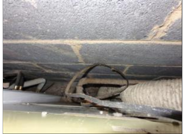
9.2 Picture 2 connection behind dryer
