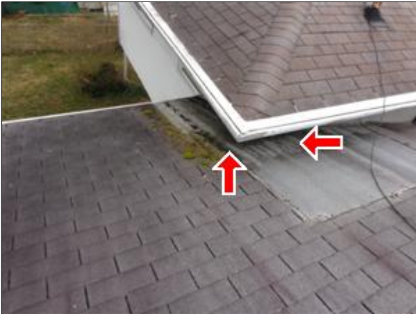
1.0 Picture 6 water can get trapped under eave
