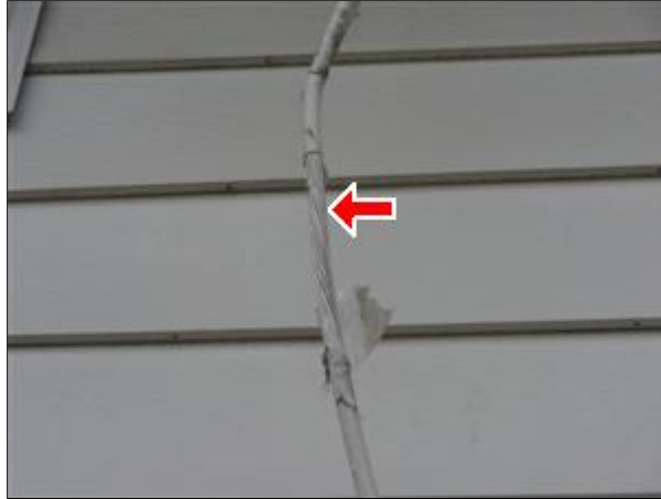
7.0 Picture 1 wires frayed here
