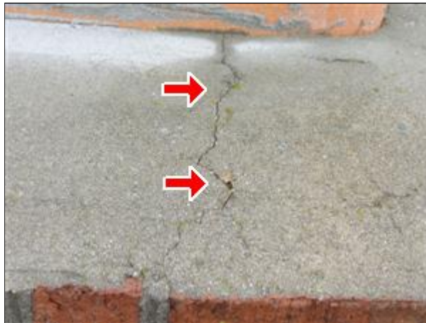
1.2 Picture 1 fill these voids
