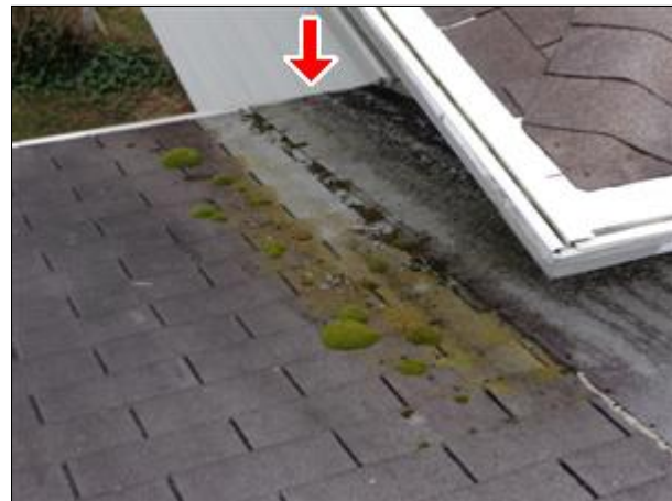
1.0 Picture 7 patch work here
