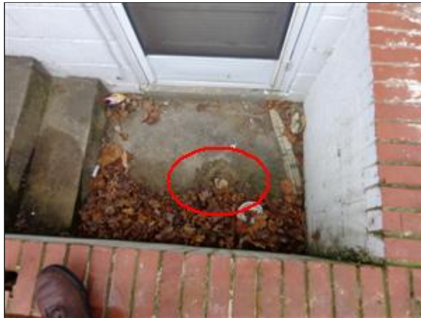
2.3 Picture 2 drain here
