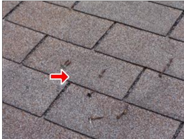
1.0 Picture 12 loose nails on roof
