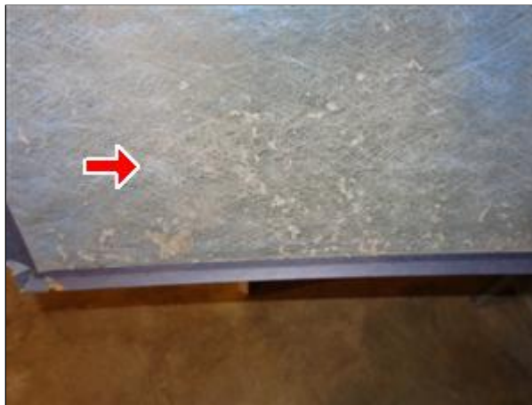
8.1 Picture 1 filter dirty
