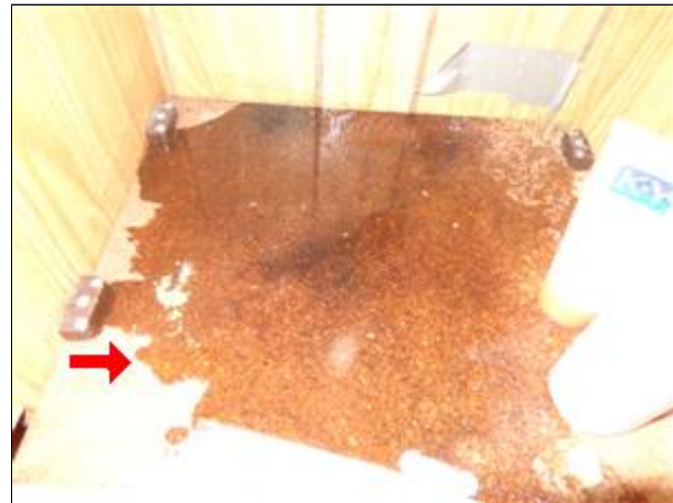
6.7 Picture 2 water leak from testing drain
