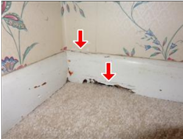
4.1 Picture 1 termite damage to trim
