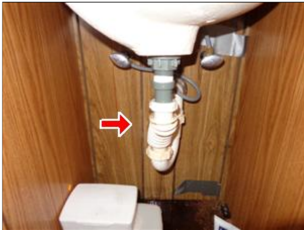
6.7 Picture 1 leaks here
