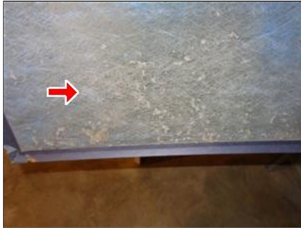
8.1 Picture 1 filter dirty
