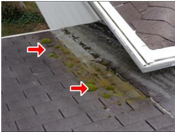
1.0 Picture 8 remove fungus on roof surface
