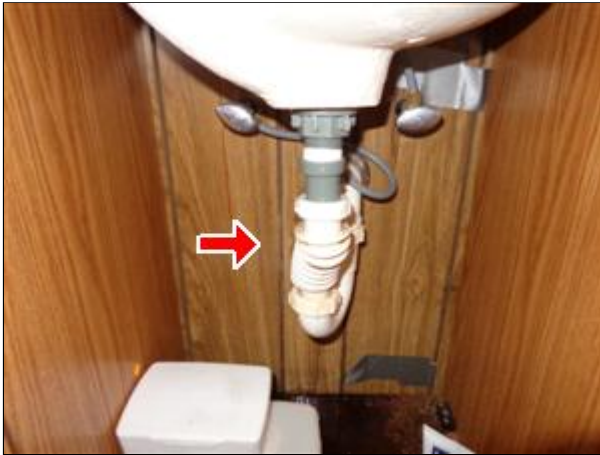
6.7 Picture 1 leaks here
