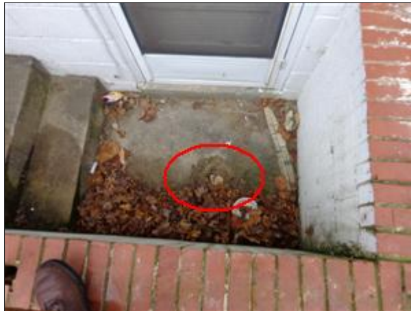
2.3 Picture 2 drain here
