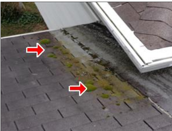
1.0 Picture 8 remove fungus on roof surface
