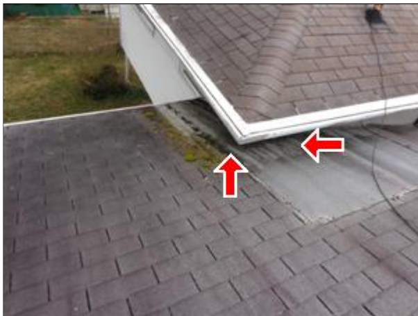
1.0 Picture 6 water can get trapped under eave
