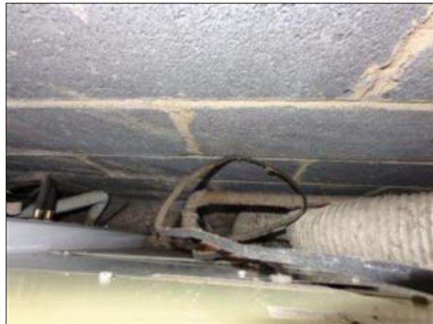
9.2 Picture 2 connection behind dryer
