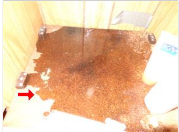
6.7 Picture 2 water leak from testing drain
