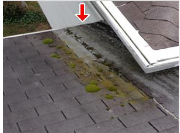
1.0 Picture 7 patch work here
