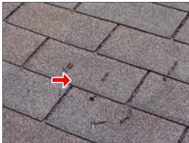
1.0 Picture 12 loose nails on roof
